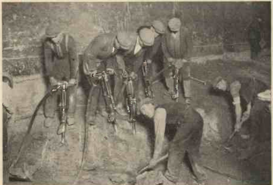
A battery of pneumatic concrete breakers in action. These five machines will break out from ten to fourteen times more material in a day than would be possible by manual labour only.
