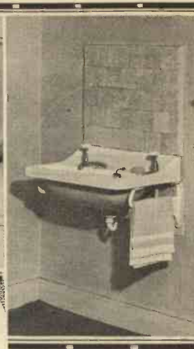
On the left is shown the method of connecting the pipe to supply water for the basin shown above. An amateur fitted this basin in a week-end at a total cost of £5 18s.
