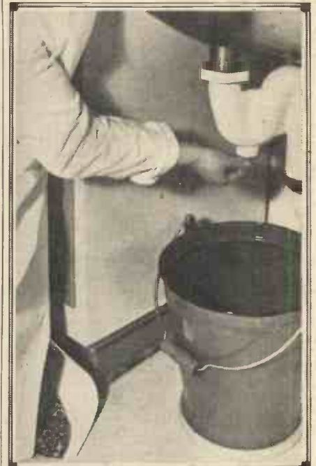
The lead trap which is fitted to all sinks, basin, and baths provides a means of catching solid matter which would otherwise pass into the waste pipe.
