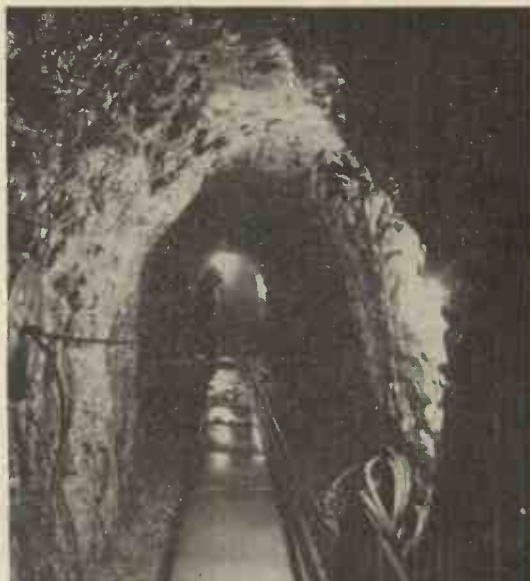
A tunnel in the chalk of North-west London to provide increased supplies and storage reservoirs. The photo was taken 300 ft. below the surface.
