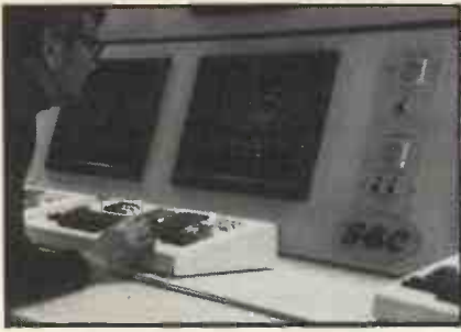
Automatic train control work station at London Docklands Light Railway Operating Centre
