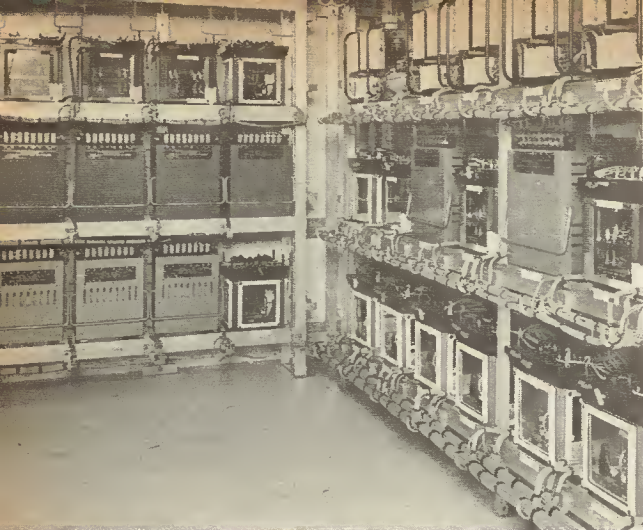
Some of the relay equipment for transmitting instructions to the trains
