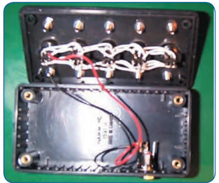
Wiring to the rear of the junction box 6-pin DIN sockets
