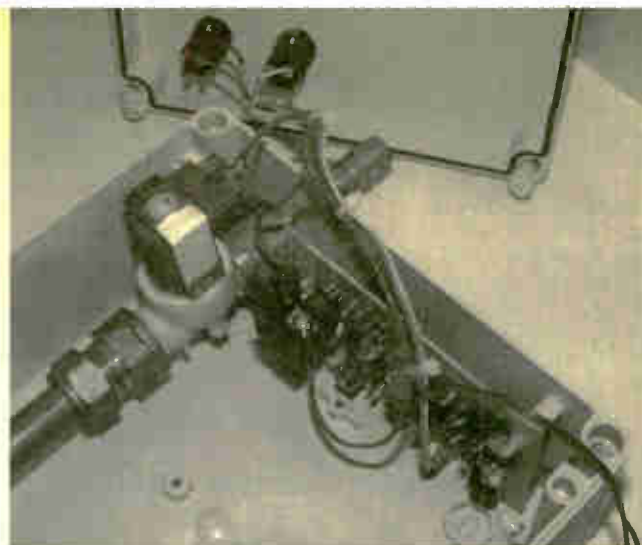
The low-voltage d.c. solenoid water valve unit mounted in one corner of the waterproof case.
