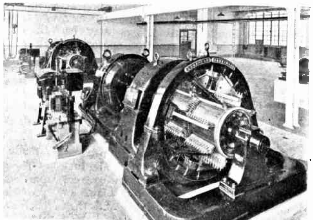
Fig. 25.—MOTOR GENERATORS FOR BATTERY CHARGING.
