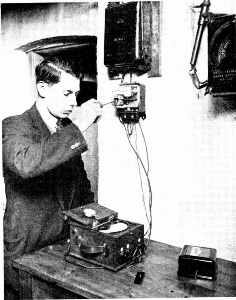
Fig. 7. —ADJUSTING THE MAGNET POSITION OF AN ARON METER AFTER CHECKING ITS PERFORMANCE WITH A PORTABLE WATTMETER AND STOP WATCH.
