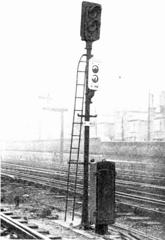
Fig. 2.—COLOUR LIGHT SIGNAL, FOG REPEATER AND TRACK CIRCUIT APPARATUS CASE.
