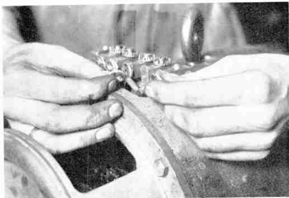
Fig. 5.—CHANGING OVER THE FIELD WINDINGS WHEN THE MOTOR RUNS IN THE WRONG DIRECTION. (Lancashire Dynamo and Crypto, Ltd.) See page 770.
