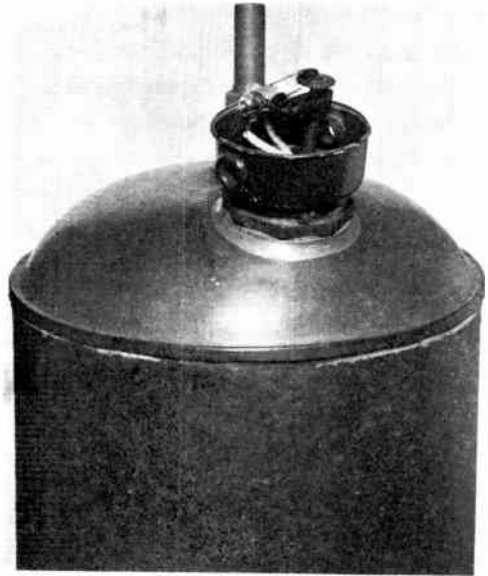
Fig. 16. —AN IMMERSION HEATER FITTED IN THE CYLINDER OF A HOT-WATER SYSTEM.
