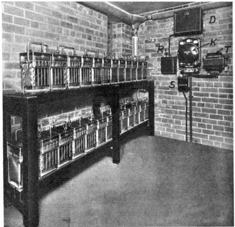
Fig. 1.—TYPICAL INSTALLATION OF SAFETY LIGHTING SUPPLY EQUIPMENT ("KEEPALITE" SYSTEM) AT A PROVINCIAL CINEMA. (Chloride Electric Storage Co.)
