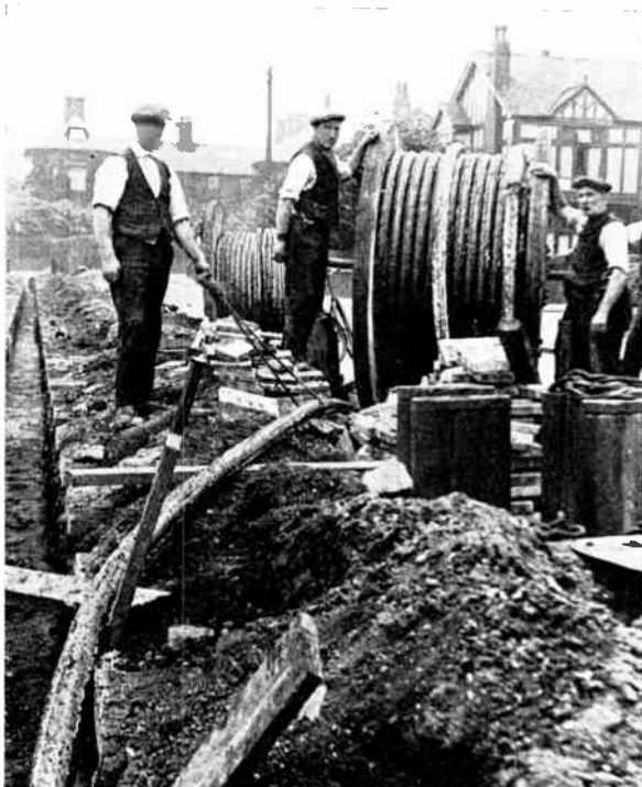
FEEDING A .5—.25—.5 SQ. IN. LOW TENSION THREE-CORE ARMOURED LEAD-COVERED CABLE IN TRENCH.
