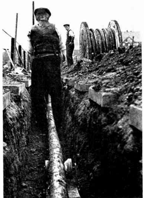
DRAWING A .5—.25—.5 SQ. IN. THREE-CORE LEAD-COVERED AND ARMOURED LOW TENSION CABLE ALONG CABLE TRENCH, SUPPORTED BY ROLLERS.
