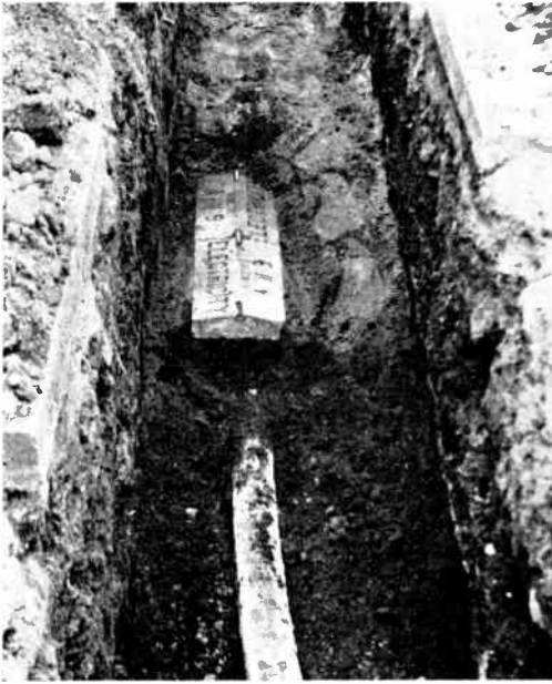
PARTIALLY FILLED-IN CABLE TRENCH.
