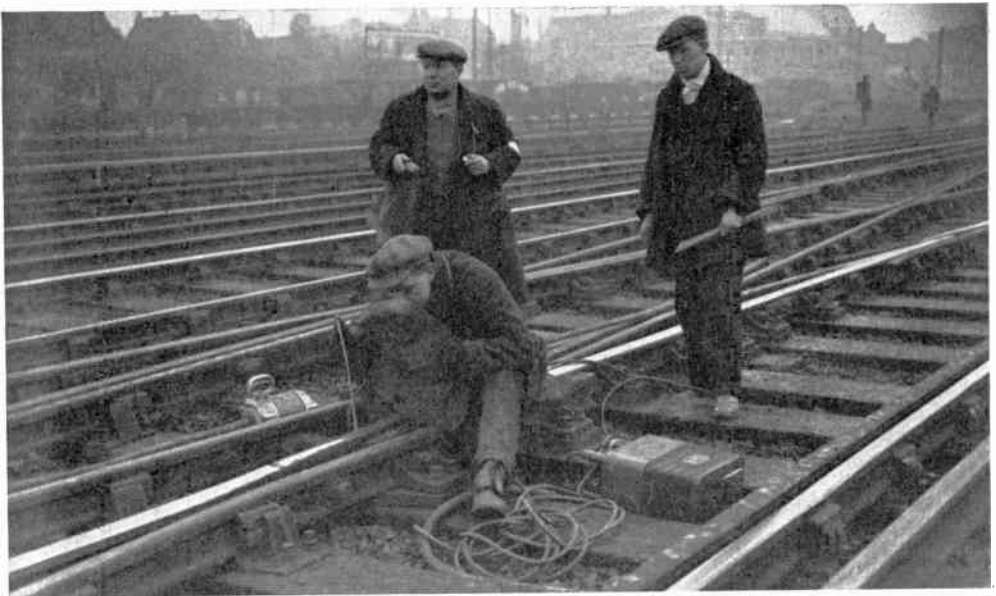
AN IMPORTANT APPLICATION OF ELECTRIC WELDING IS THE REPAIR OF RAILWAY TRACK. This shows a welding operator in position, ready to strike the arc.
