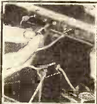
It is often a good plan to support the G.B. battery under the lid of the cabinet, as shown.
