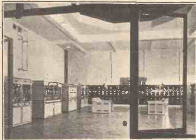
The main transmitter hall, showing the two control desks at which the engineers will sit whilst the twin stations are working.
