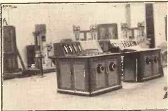
These are the principal switchboards for control work, their neat exteriors hiding a complicated mass of connections.
