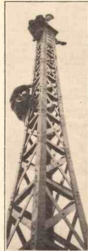
Workmen on one of the masts above the new home of the B.B.C. in Portland Place.
