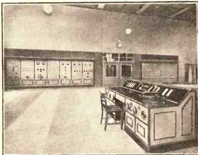
The engineer-in-charge at Heilsberg can switch on the transmitter and control the whole transmission from this desk.
