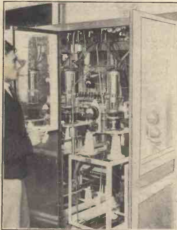
A Marconi engineer examining one of the main panels of the new 160 kw. broadcaster to be erected near Warsaw. It will be the most powerful broadcasting station in Europe.
