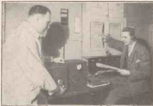
The amplifier room at the Berlin Opera House which is frequently "on the air."
