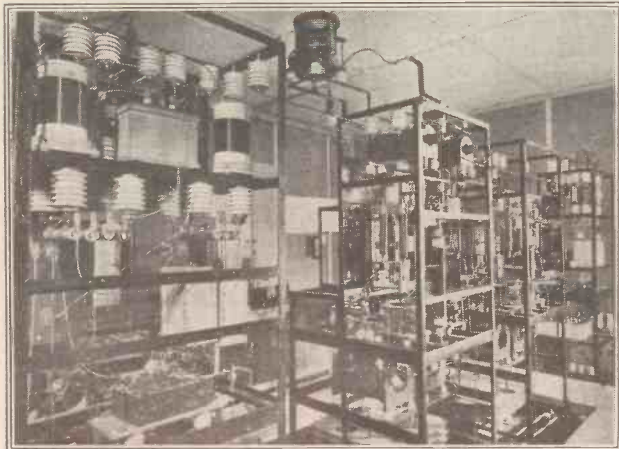
The transmitting apparatus at the new Rome broadcasting station.
