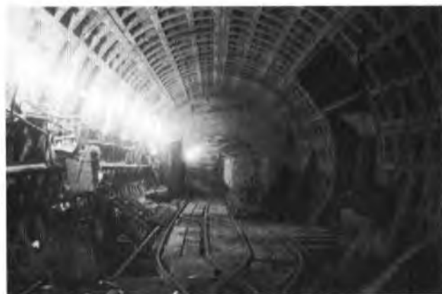
FIG. 6—The main enlargement (the west tunnel junction can be seen on the right-hand side of the photograph)
