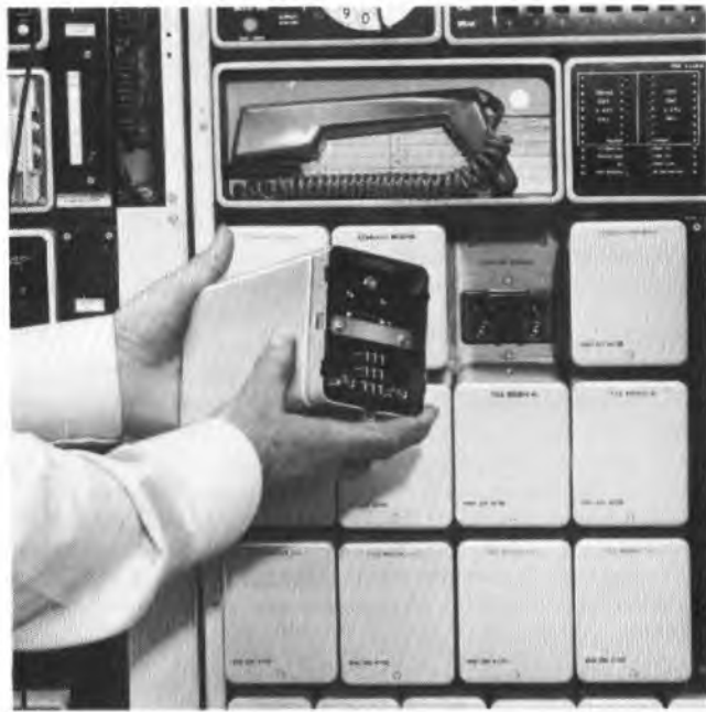
FIG. 6—A unit removed from a conclave rack
