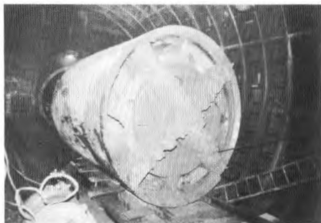
FIG. 4—Digger shield (at the end of its drive) showing the cutting face
