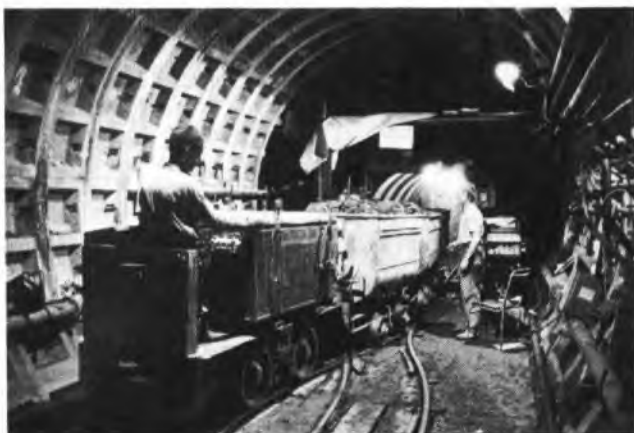
FIG. 7—Chamber at the foot of the work shaft with a train of skips leaving the air lock
