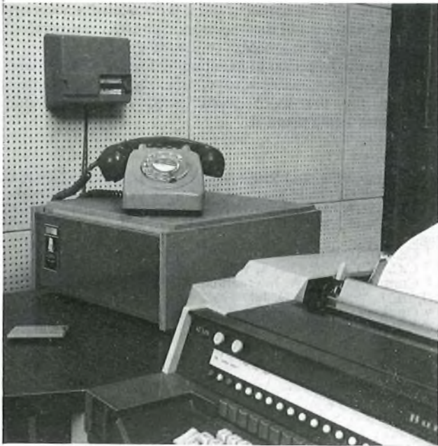
FIG. 3—Outstation showing Case No. 200, modem, standby telephone and the customer's terminal
