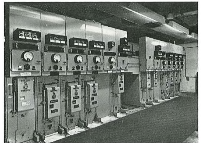
FIG. 1—Thirteen-panel high-voltage board in Mount Pleasant sub-station
