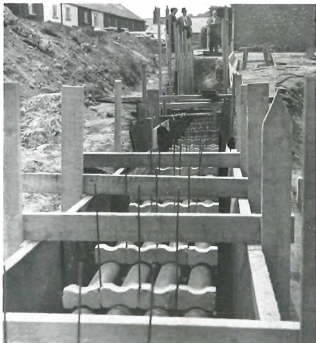
DUCTWORK AT KNUTSFORD TELEPHONE EXCHANGE
