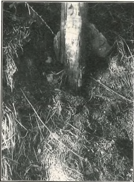
POLE DAMAGED BY LIGHTNING STRIKE.
