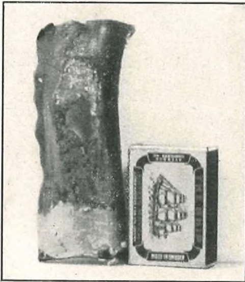
DAMAGE DONE TO CABLE SHEATH BY DORMOUSE.
