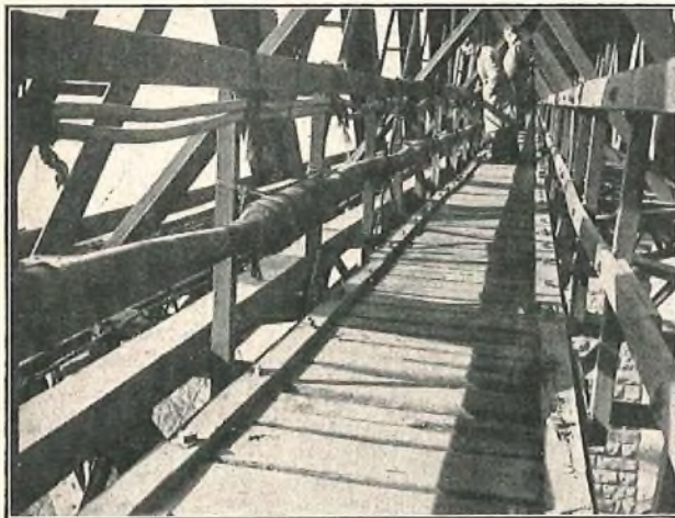
FIG. 4.—INTERRUPTION CABLE ON CATWALK.
