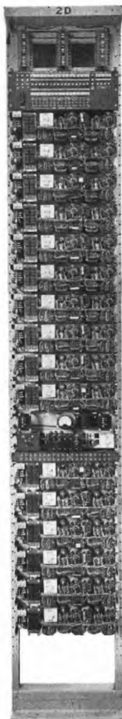
Bay mounting 2-wire Voice-frequency Repeater Equipment with covers removed
