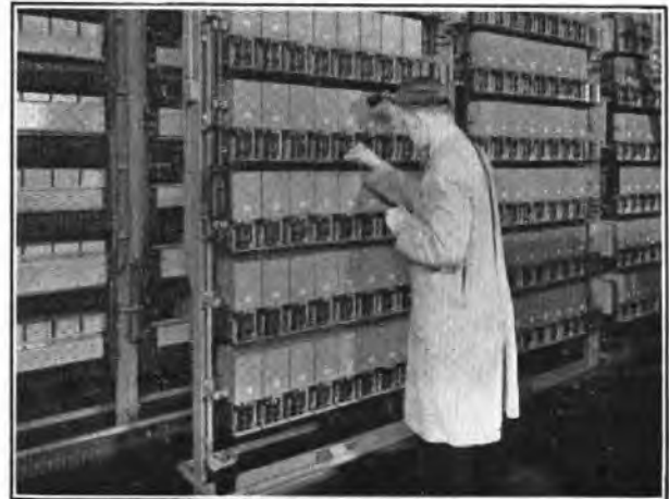
COMPLETED AUTOMATIC EXCHANGE IN SERVICE.
