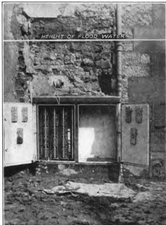
CABINET AFTER SUBMERSION BY FLOODS.
