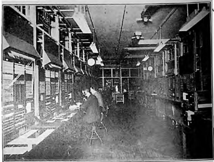
FIG. 3.—TRUNK TEST RACKS IN CITADEL.
