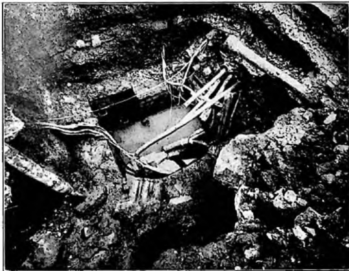
FIG. 4.—DAMAGE TO UNDERGROUND PLANT (BRIXTON, LONDON)
