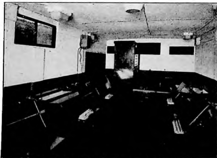
FIG. 6.—INTERIOR OF MOBILE TELEPRINTER ROOM.
