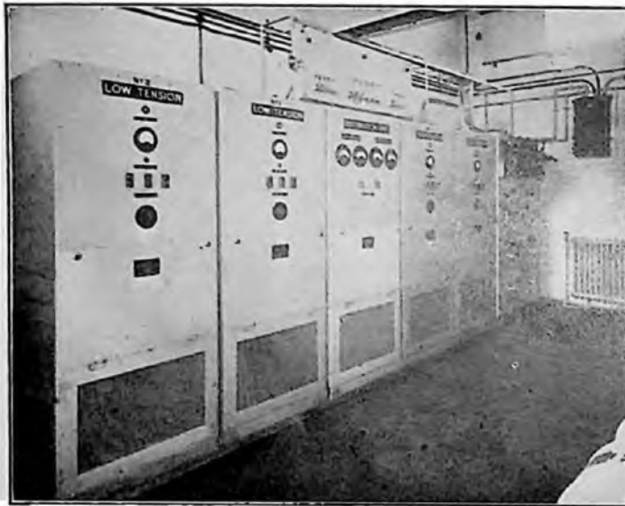
FIG. 3.—POWER PLANT FOR D.T.N. STATION.
