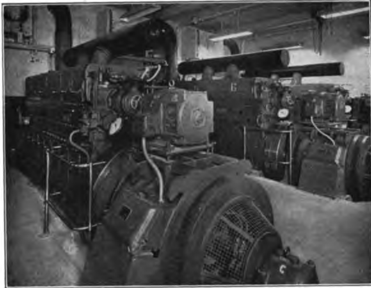
FIG. 3.—GENERAL VIEW OF PLANT.
