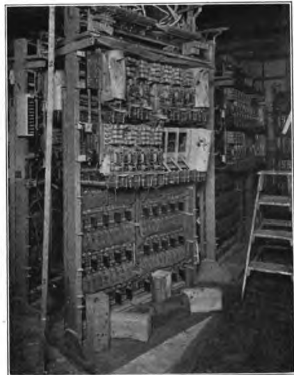
FIG. 3.—DAMAGE TO AUTOMATIC EQUIPMENT BY H.E. BOMB.
