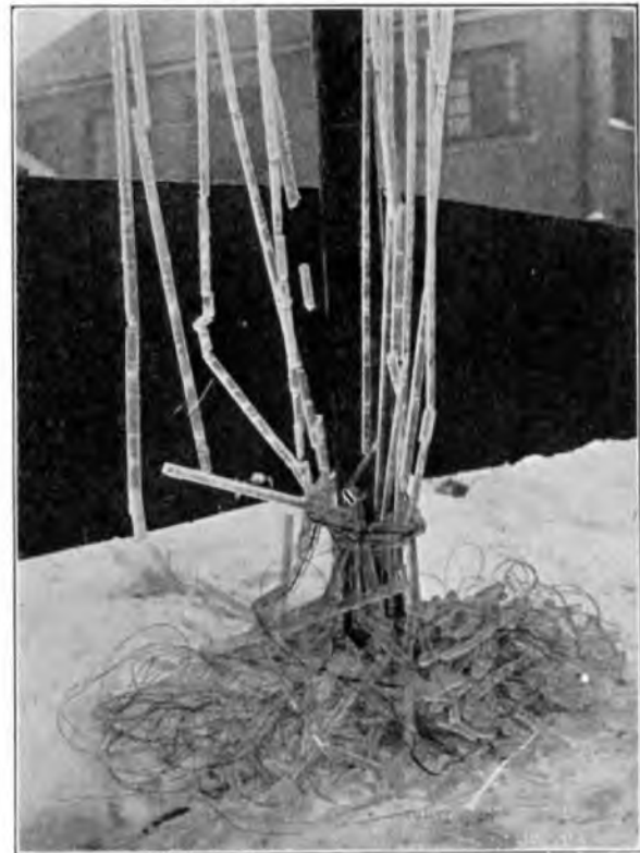
FIG. 10.—ICE-COATED WIRES AT PORTSDOWN HILL, SOUTHAMPTON AREA.
