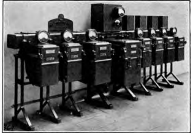
FIG. 3.—MAIN LOW TENSION SWITCHBOARD, EUSTON TELEPHONE EXCHANGE.
