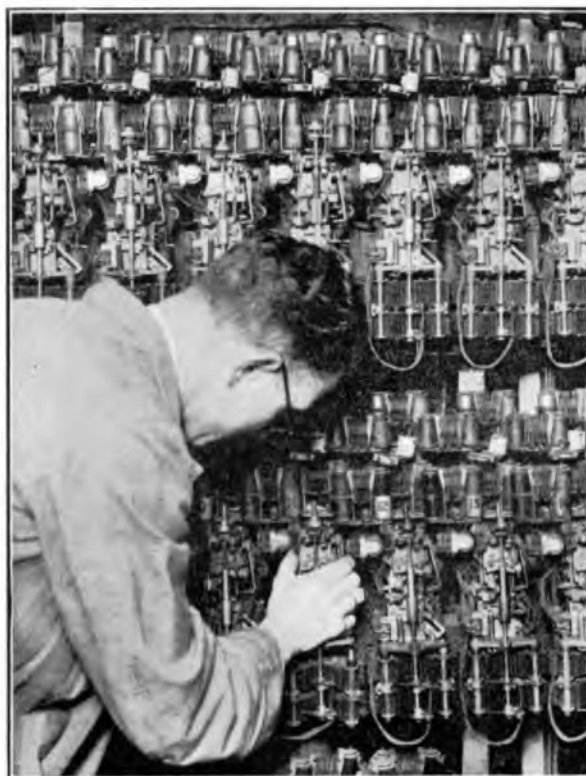
FIG. 3.—UNIT 600, SHOWING DETAILS OF FINAL SELECTORS.
