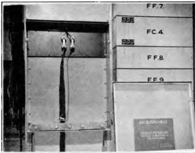
FIG. 9.—CABLE TERMINATION BAY.
