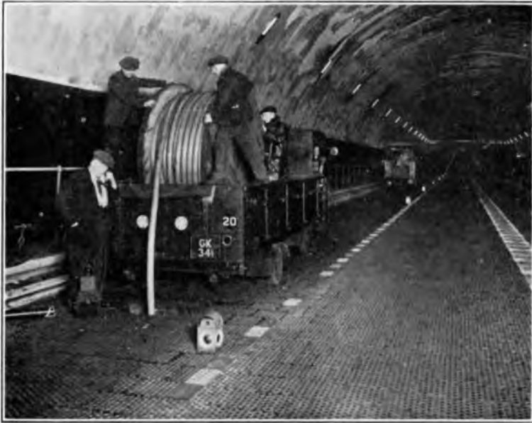
FIG. 6.—CABLING FROM TUNNEL ROADWAY.
