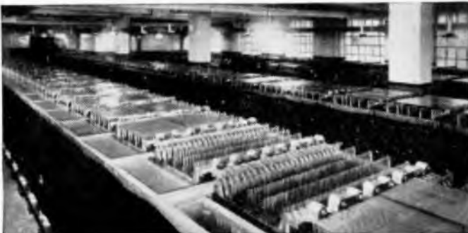
Illustration shows an installation of Alton Batteries of merit at an important London Telephone Exchange.
