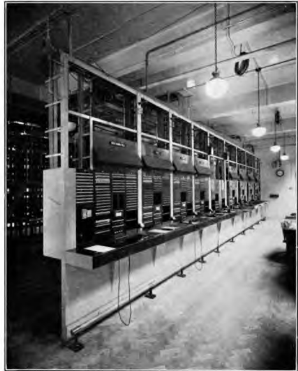
FIG. 7.—TRUNK TEST RACKS.
