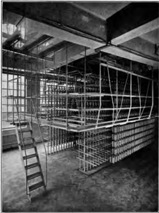
FIG. 6.—M.D.F. SHOWING MEZZANINE PLATFORM.
