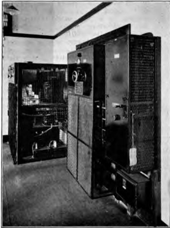
FIG. 7.—POWER SUPPLY RECTIFIERS.
