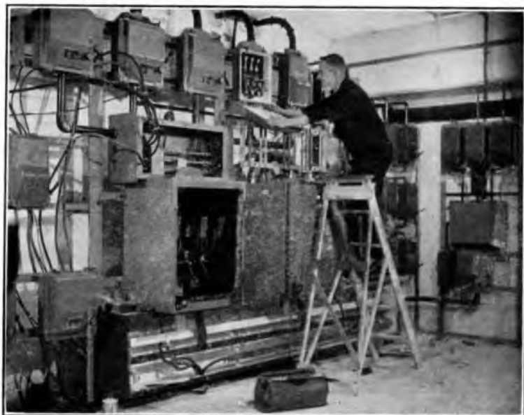
FIG. 5.—DEPARTMENT'S L.T. SWITCHBOARD.
