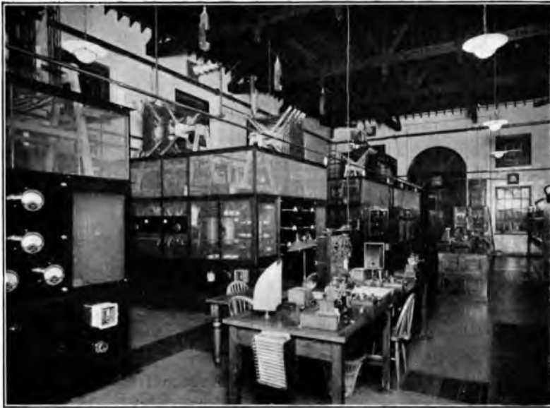
FIG. 2.—MAIN TRANSMITTING ROOM.
