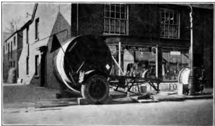
FIG. 3.—CABLING AT FOOTWAY JOINT BOX.
