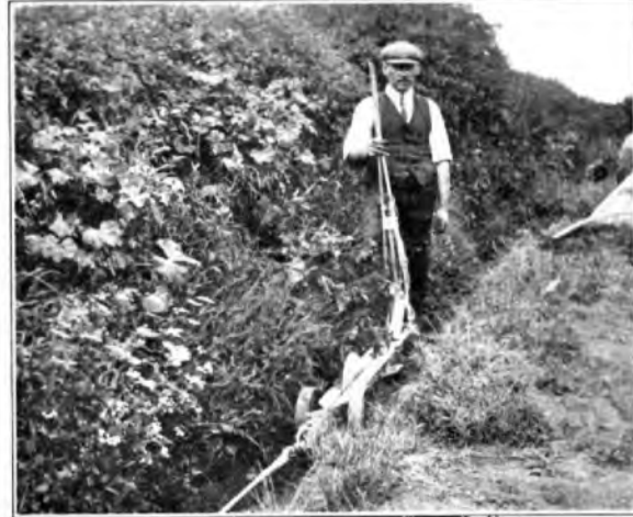
Fig. 11.—Small Mole Drainer in action in ploughed furrow. Note cable entering joint hole.
