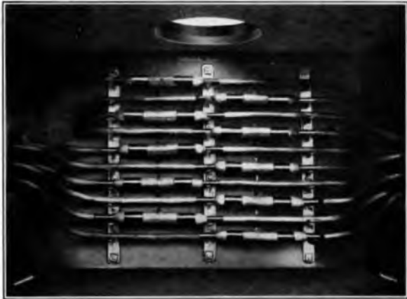
FIG. 3.—PHOTOGRAPH OF PORTION OF A MODEL MANHOLE WITH CABLES AND JOINTS SUPPORTED ON SIDE WALLS.
