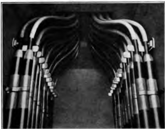
FIG. 5.—PHOTOGRAPH OF PORTION OF A MODEL MANHOLE WITH CABLES AND JOINTS SUPPORTED ON SIDE WALLS.
