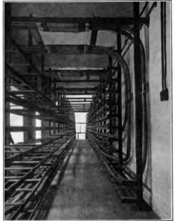
FIG. 10.—PHOTOGRAPH OF LEADING IN ARRANGEMENTS, NEWCASTLE CENTRAL AUTOMATIC EXCHANGE.
