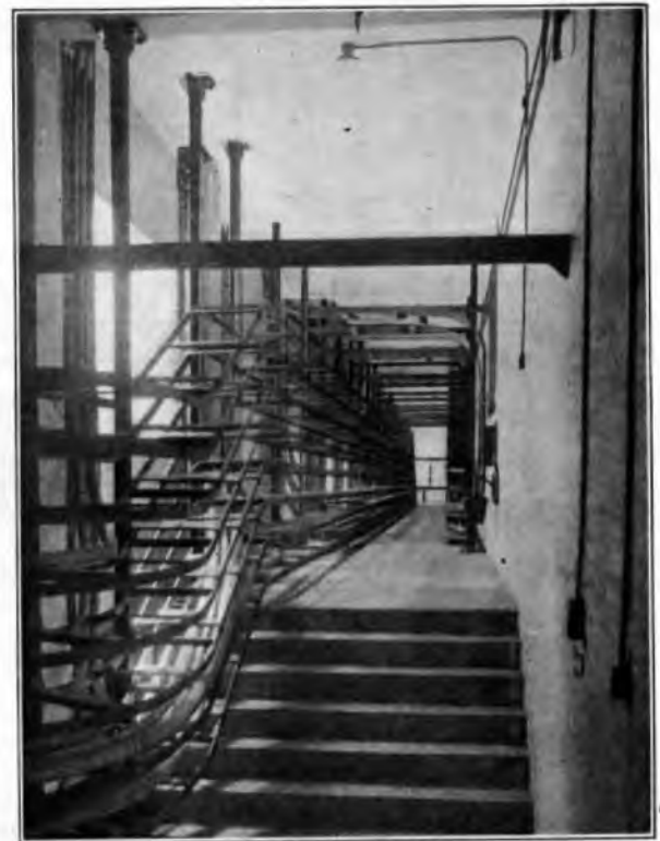
FIG. 11.—PHOTOGRAPH OF LEADING IN ARRANGEMENTS, NEWCASTLE CENTRAL AUTOMATIC EXCHANGE.
