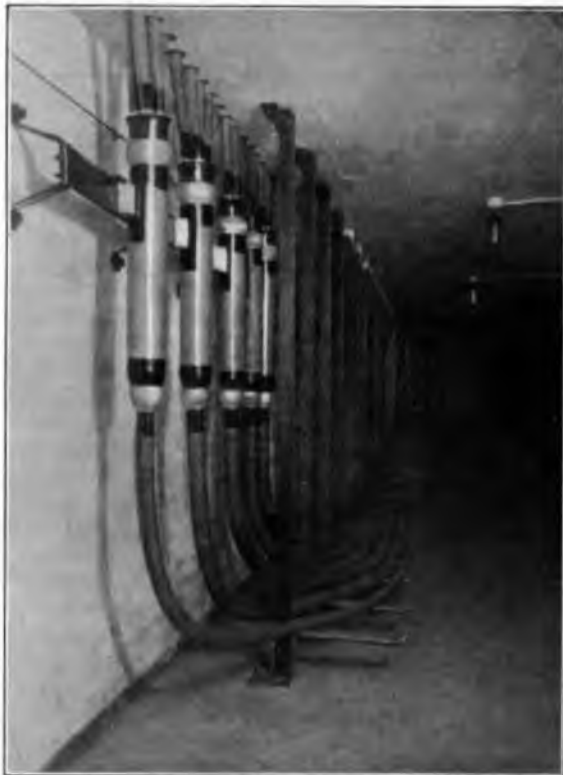
FIG. 7.—PHOTOGRAPH OF LEADING IN ARRANGEMENTS, NEWCASTLE EAST EXCHANGE.
