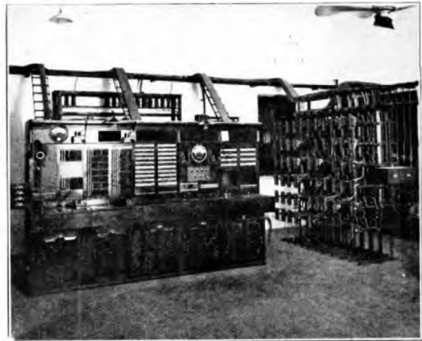
FIG. 6.—TEST ROOM, NEW DELHI. Shows Test and Morse Board, incoming Cables, M.D.F. and Composite Apparatus Rack.
