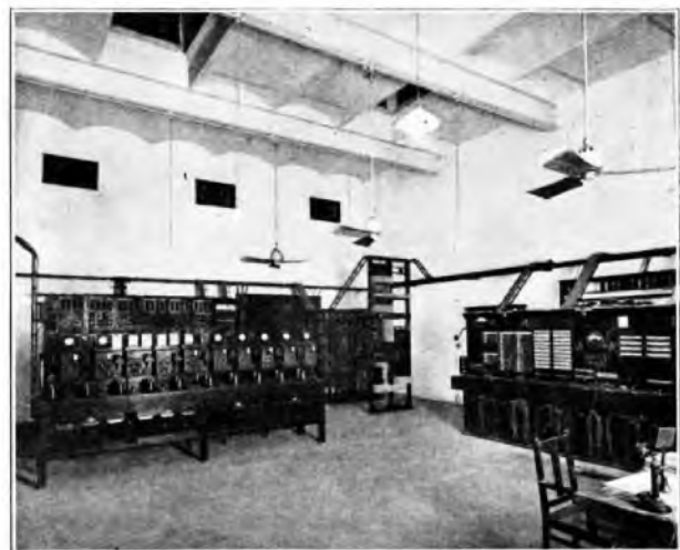
FIG. 7.—TEST ROOM, NEW DELHI. Shows Test and Morse Board, Duplex Sets, Cord Circuit Repeater, Battery Tap Rack and I.D.F.
