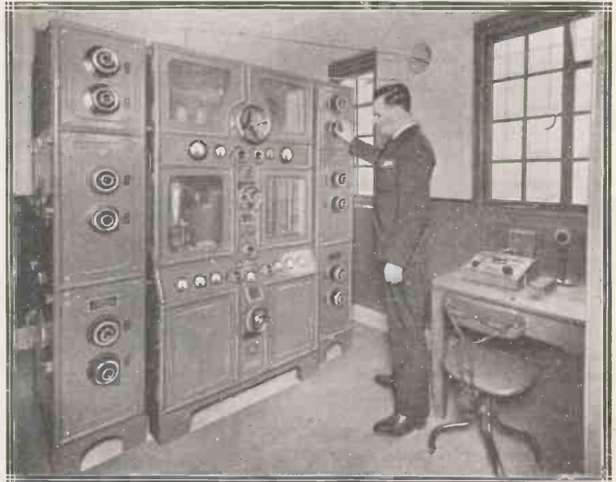
Manufactured, designed and installed by the Marconi Company, this magnificent transmitter places Manchester's air port among the most efficiently equipped in the country. The circuit comprises master oscillator, one stage of power amplification, and a coupled aerial circuit.
