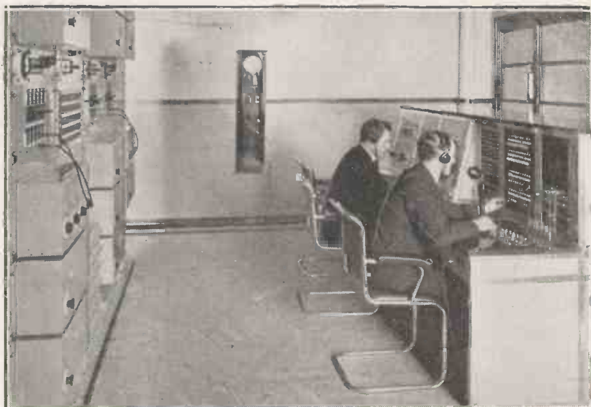
The control room at the new Leeds studios is a replica in miniature of the main control room in London. Here we see two of the control desks together with a portion of the amplifying equipment.
