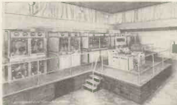
On a raised platform will be seen the transmission panels and control desk of Schweizerischer Landessender, the Swiss transmitter which uses a power of 60 kilowatts on 459 metres.
