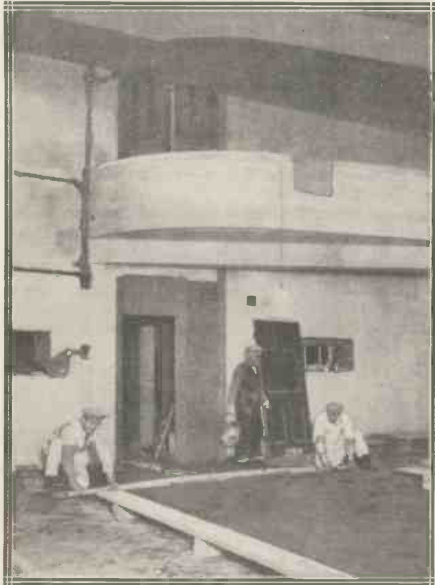
Workmen cementing the gallery floor of the giant studio in the B.B.C.'s Portland Place headquarters.
