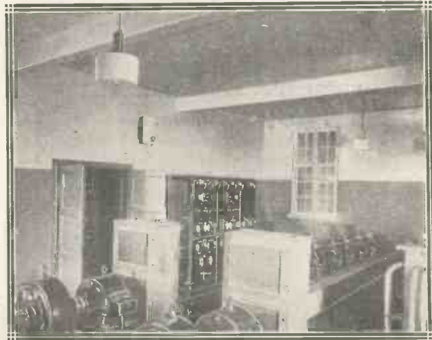
The large generators are housed in a separate room, well away from the actual transmitting gear.
