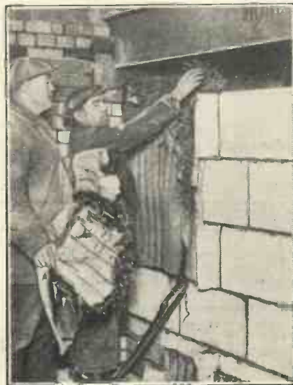
Very thick seaweed-lined cellular concrete walls are being used at Broadcasting House to render the studios immune from outside noises. The photo shows workmen placing the seaweed in position.
