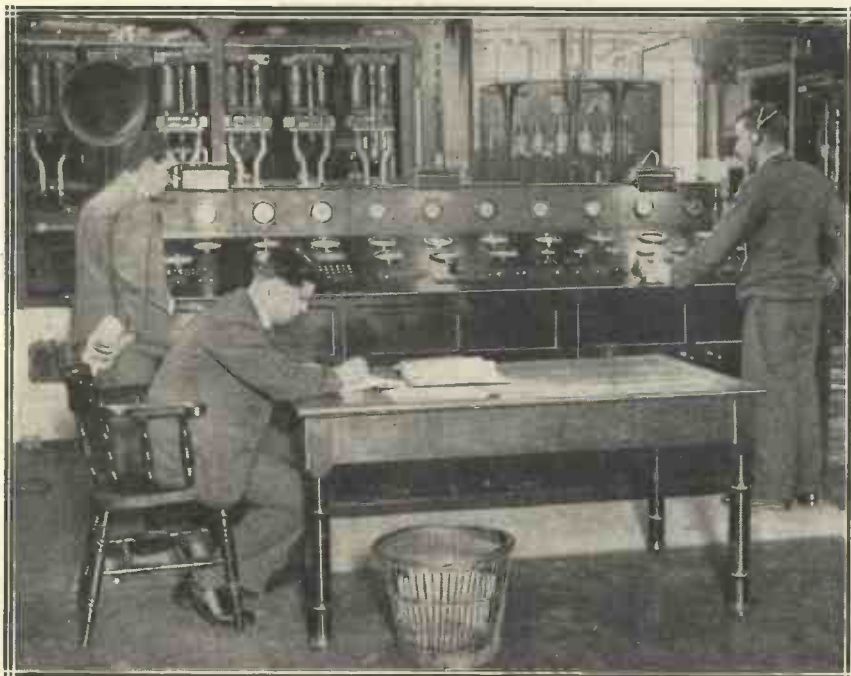
The control-room of the long wave transatlantic telephony section of the Rugby station. All telephonic communication between this country and the U.S. goes through this gigantic radio nerve-centre.
