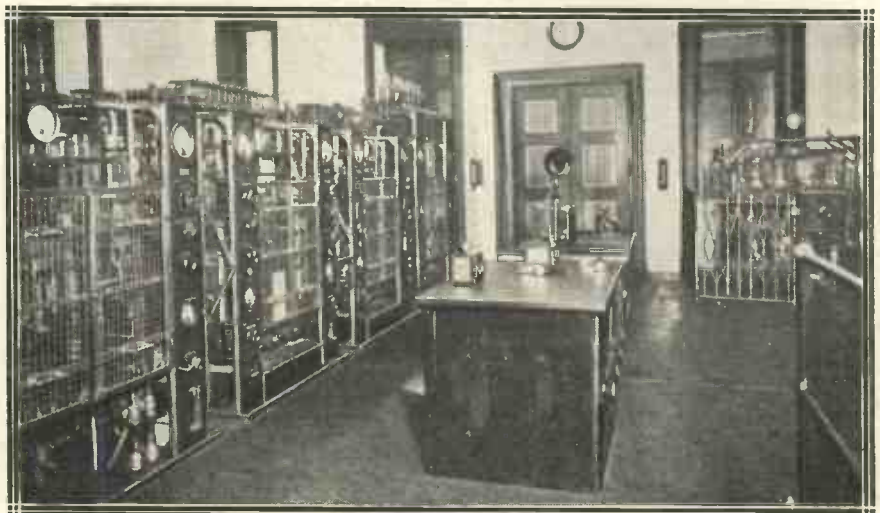
Very carefully-thought-out screening has to be employed in big transmitting stations. Here we see the interior of the power-house at the Vatican.
