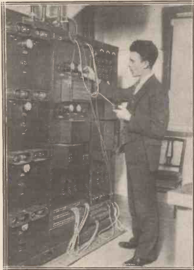
This is the control room of the Pennsylvania Hotel's radio system. Every room has a connection, and guests can choose their own individual station. Over 33 million feet of wire were used for this system in the great New York hotel.
