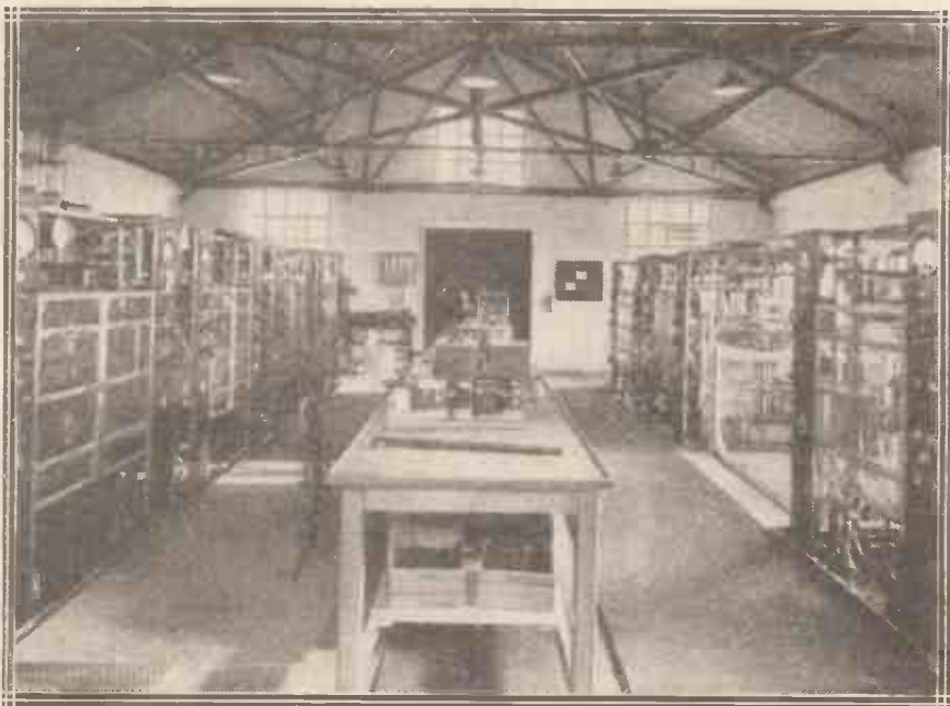
This is the transmitter room of the Marconi Short-Wave Beam Wireless transmitting station at Dorchester. The transmitter on the left is used for communication with New York on three wave-lengths and the transmitter on the right is used for working with Rio de Janeiro on one wave-length.
