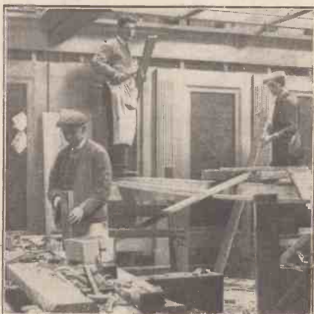
Work is proceeding apace in the building of new studios at the Belfast station. Above can be seen one of the smaller studios in the course of construction. This is to be used for talks and chamber music. Note the echo-proof lining which is being fixed behind the panelling.
