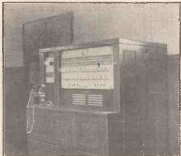
Above is shown the control switchboard, where the engineer-in-charge has all Norddeich's powerful apparatus at his finger-tips.
