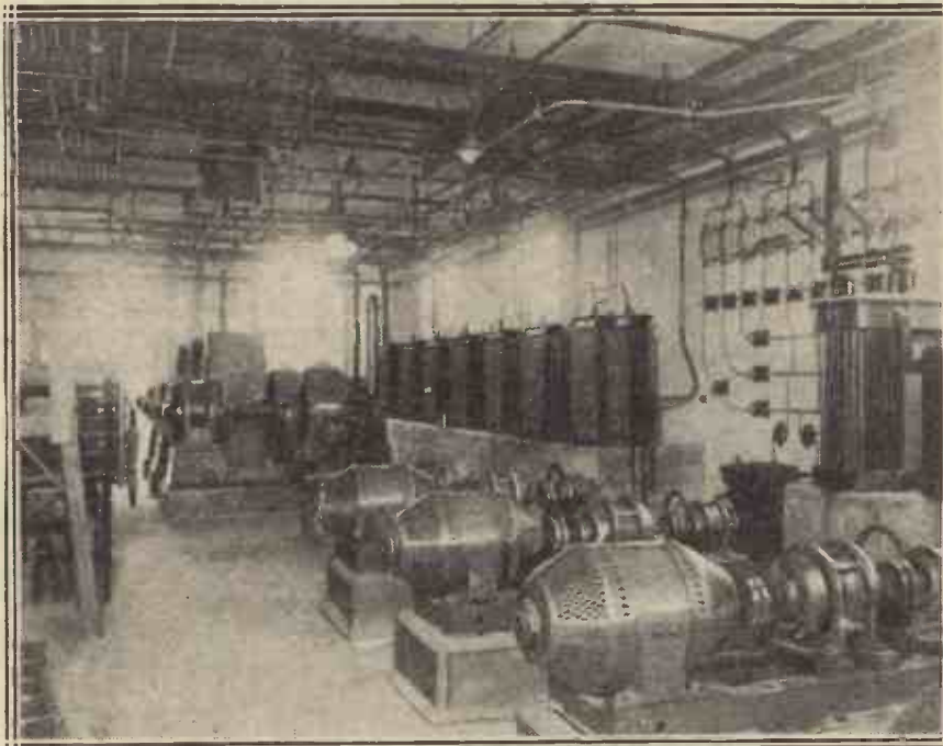
The huge motor-generator room of an American broadcasting station. W E A F's new 50-kw. plant is situated at Bellmore, L.I., N.Y.
