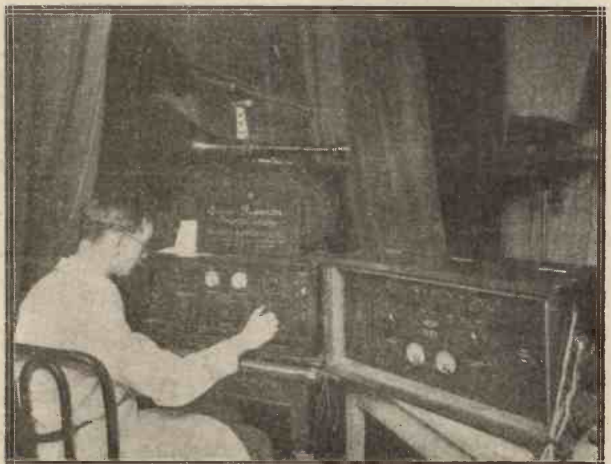
Graham Amplion public-address equipment installed at a London cinema. Animal noises were projected in synchronism with a film.
