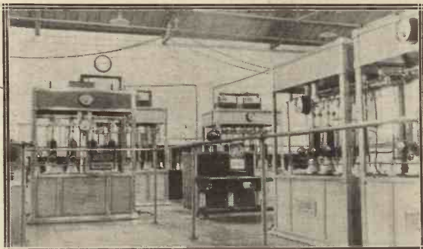
Some of the transmitter panels at 5XX. The big water-cooled valves have to be carefully looked after, as they cost £80 each.
