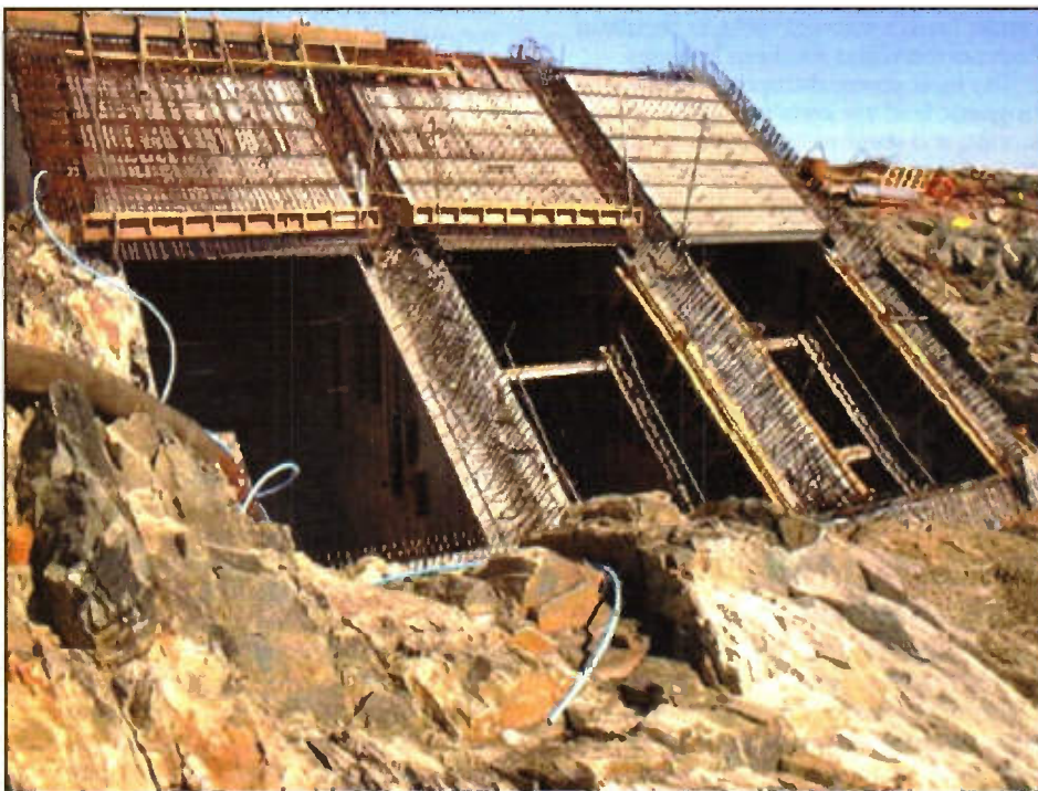
Photo 8. (islay476.jpg) Detail of cliff top construction of LIMPET 500 wave power facility (Courtesy WAVEGEN).
