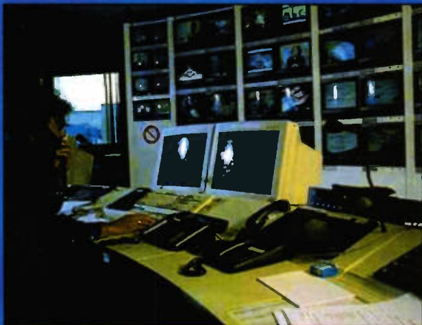
Eutelsat control room.
