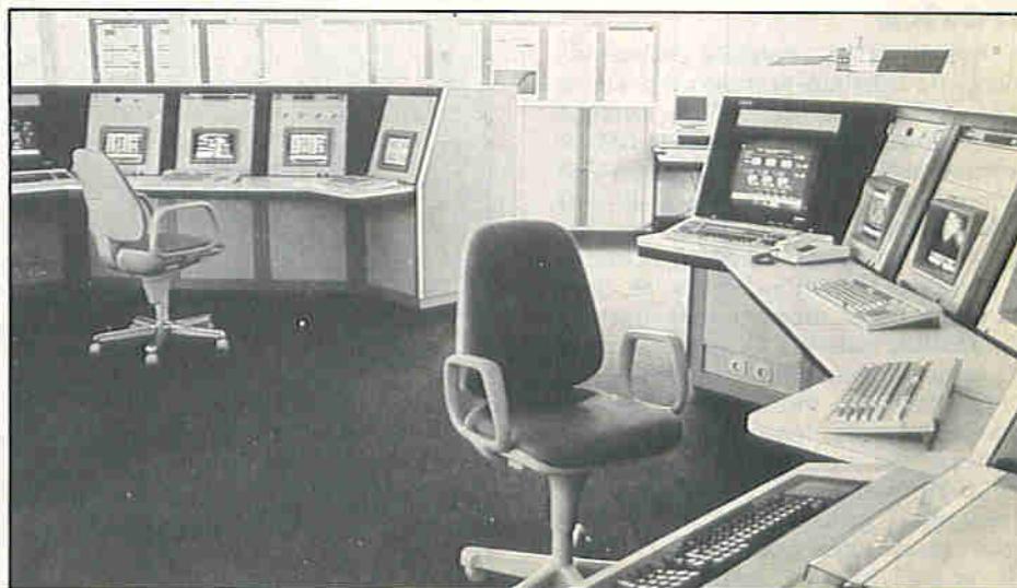
Inside the control room at Astra's Betzdorf Satellite Operations Centre.
