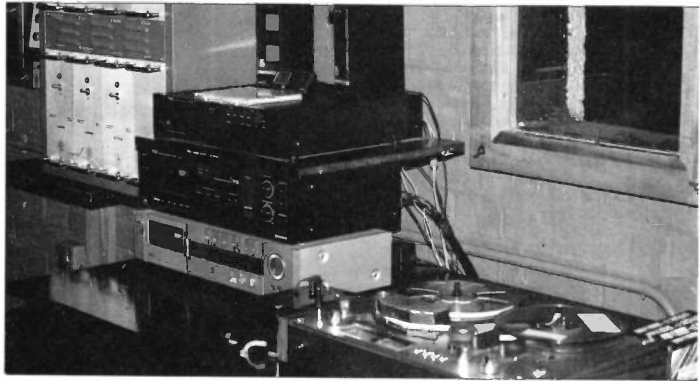
Photo 4. Audio equipment; left of centre, 6 x 200W and 1 x 100W (1.3kW) audio power amplifiers; centre, CD player and cassette recorders; right of centre, open reel tape recorder.
