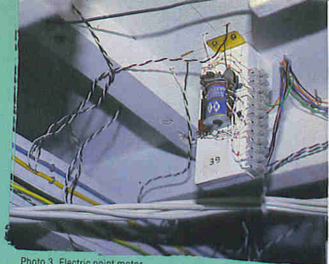
Photo 3. Electric point motor.
