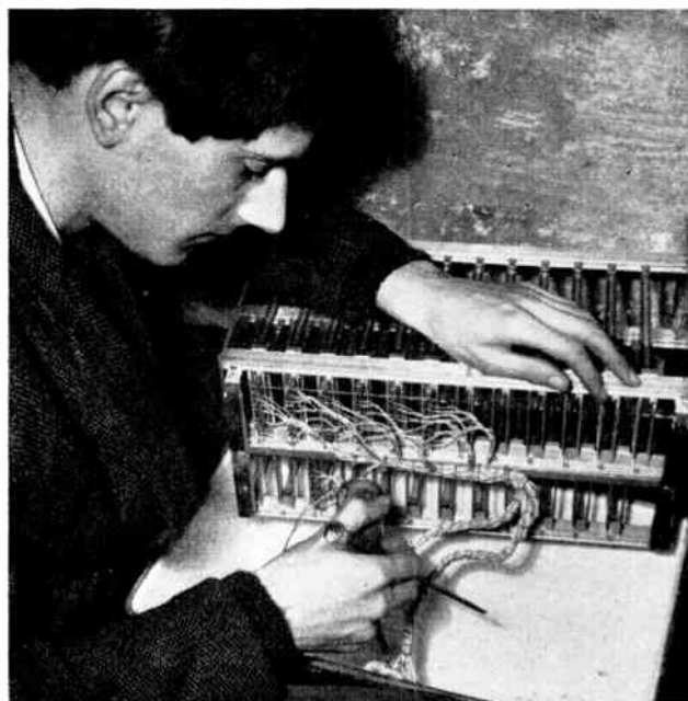
A p.c.m. repeater in a loading-coil manhole. When fully equipped this framework will hold regenerators for 24 complete systems, each of 23 two-way circuits
